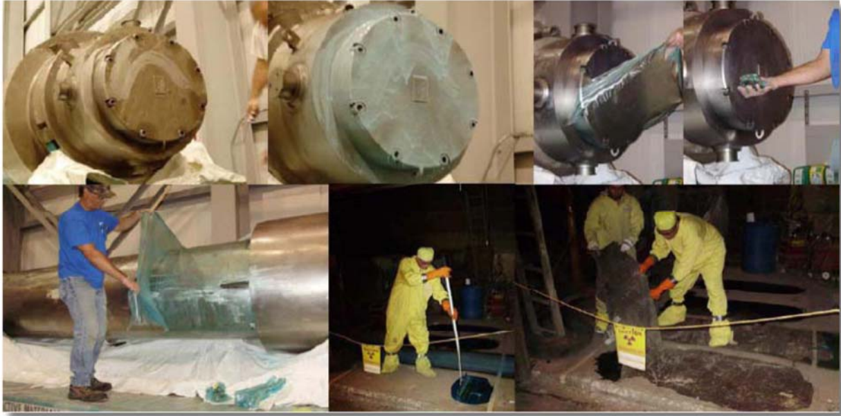
Figure 3. Decontamination field test at Alaron Nuclear Services with DG showing radioactive isotope removal from a nuclear fuel cask container and areas of a shop floor.
